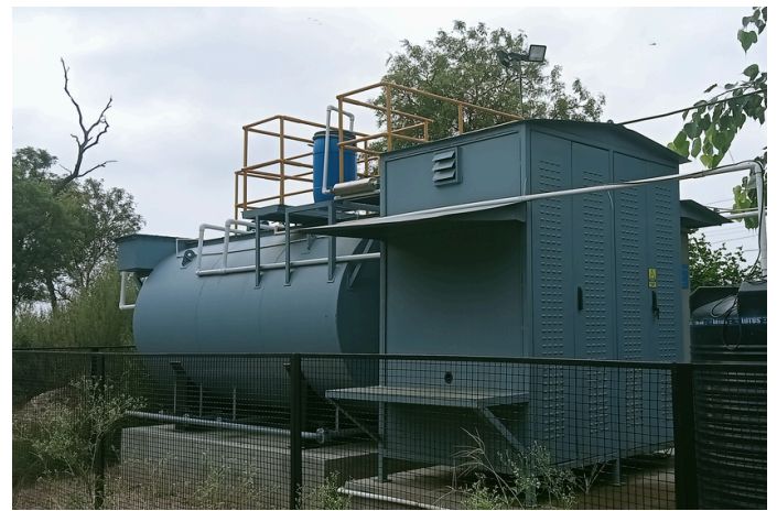
Above Ground Plant
