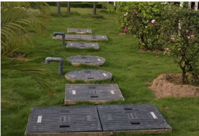
Under Ground Plant
