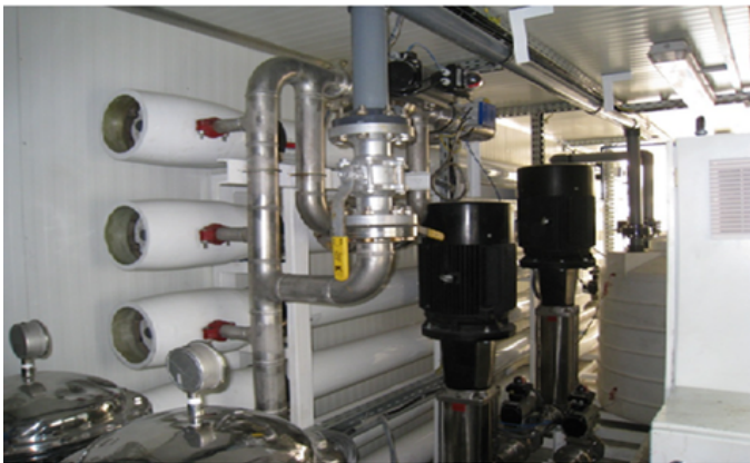
Name of Project : BWROPU for US Army Base in Iraq Capacity : 2 x 28500 LPH Year of Completion : 2007 Approving Authority : Bechtel
