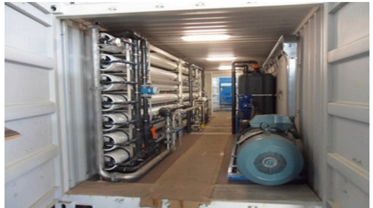
Name of Project: BWROWPU for Bagram Air Base in Afghanistan Capacity : 2 x 28500 LPH Approving Authority : Bechtel Year of Completion : 2008
